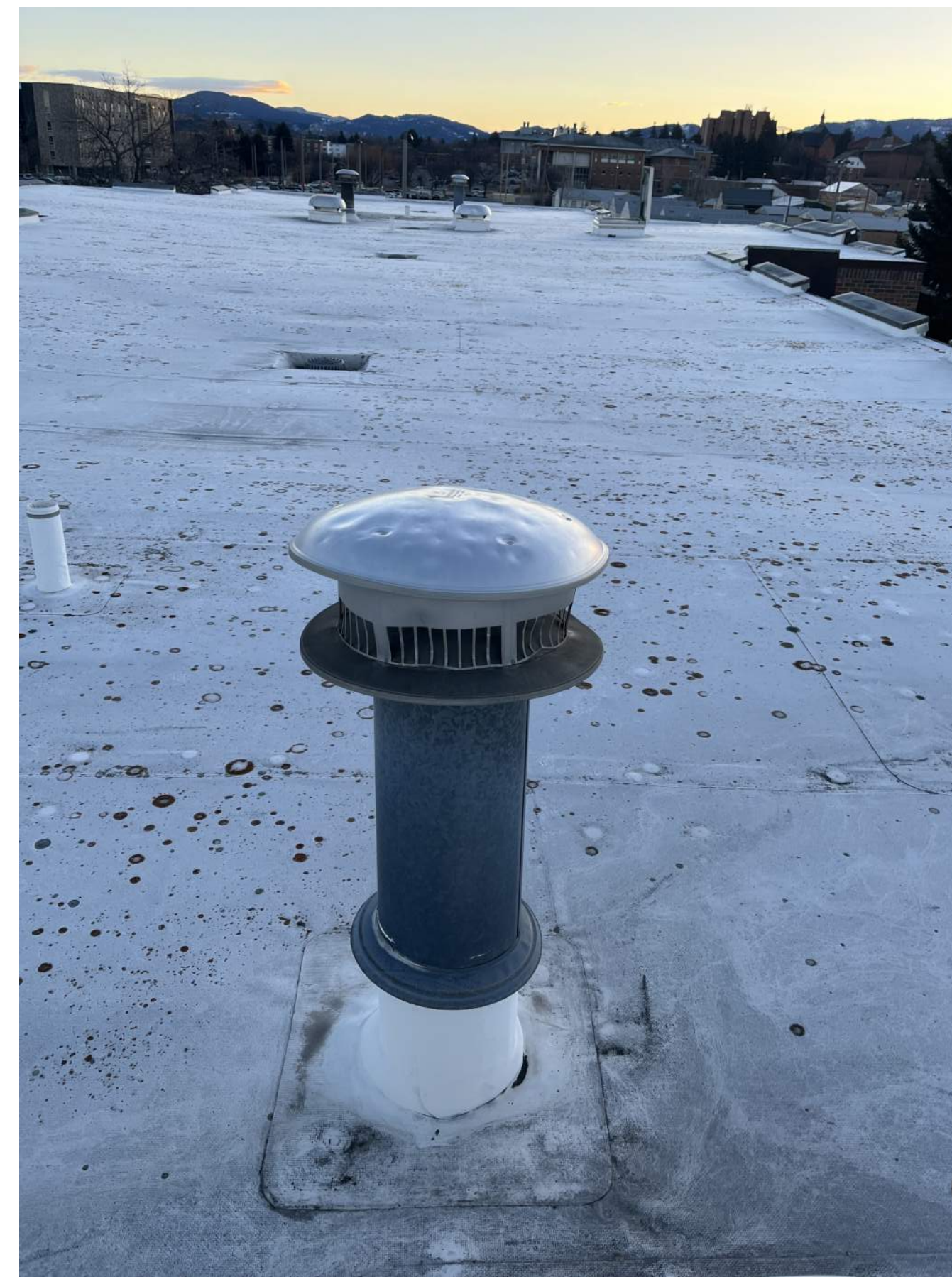
EXISTING BOILER AND/OR HOT WATER VENT, TYPICAL CONDITION.
